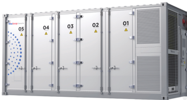
Example battery container
